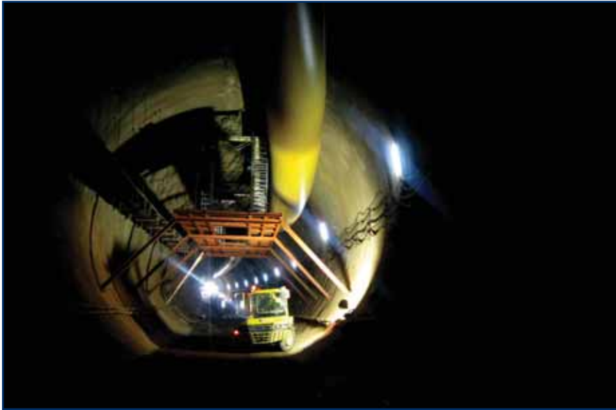
Figure 4: Dewatering Shaft Access Platform at Tunnel Low Point
