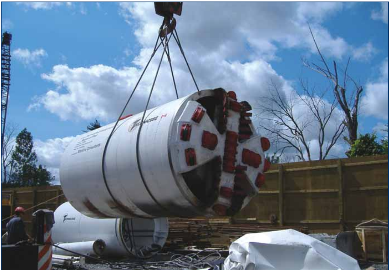
Tunnel Boring Machine (TBM) that was used to complete 2 of the 3 northerly tunnel drives. The first section of the TBM is being lowered into Shaft #1
