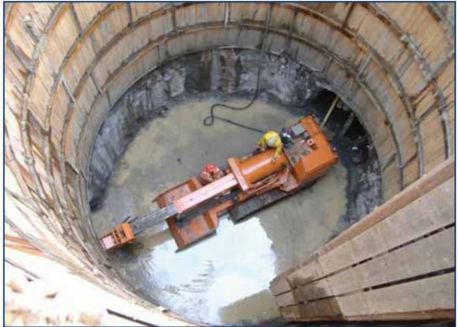
Tunnel Digging Machine (TDM) manufactured by Technicore, that was used to complete the back tunnel around a sharp curve south towards the Credit River
