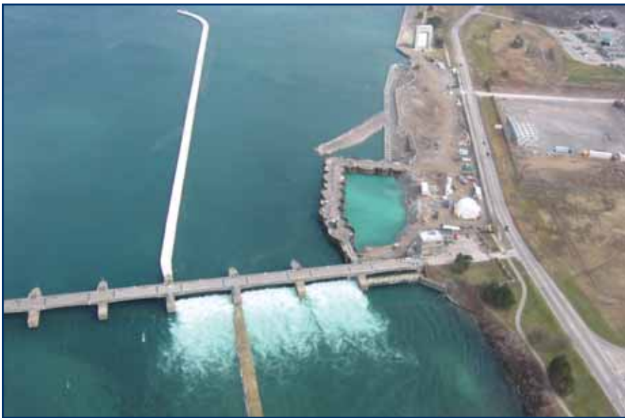
Figure 5: Aerial View of Intake Site with Cofferdam, Ice Groyne and New Accelerating Wall in Place
