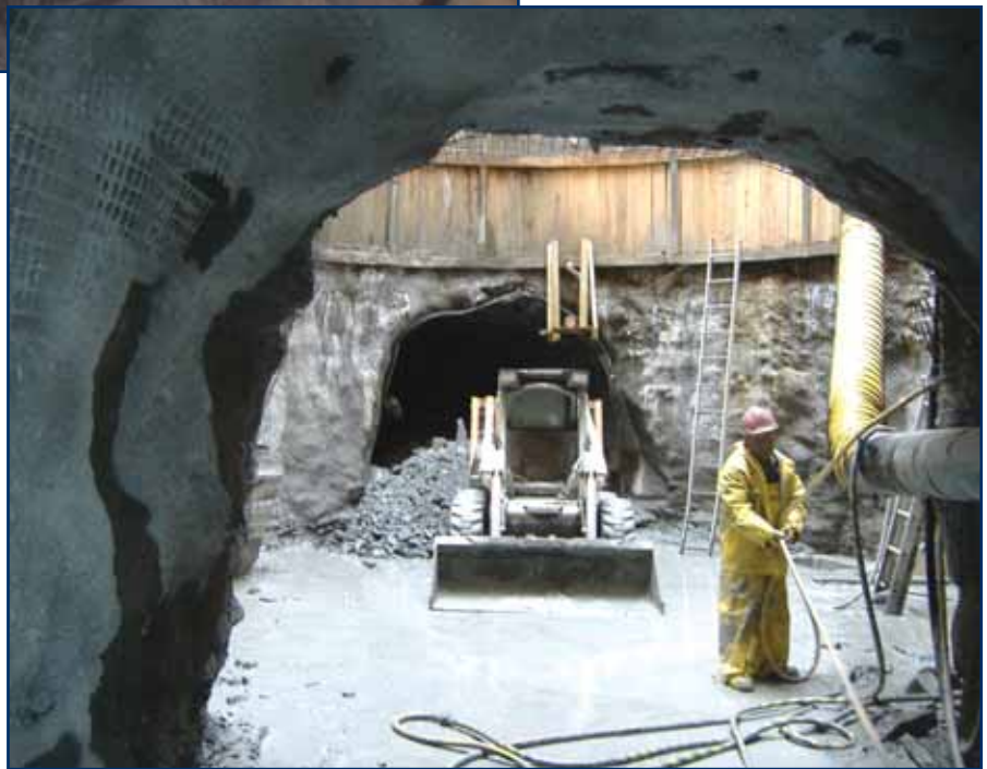
Looking south from within the horseshoe-shaped starter tunnel at Shaft #1, which was over-excavated in order to accommodate a switch
