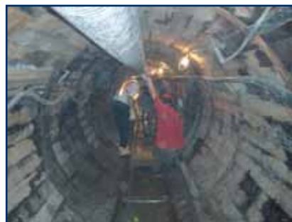
Primary tunnel liner, which was constructed of steel ribs and hardwood lagging
