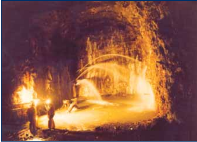
Figure 2. High-pressure water inflows in tunnel
