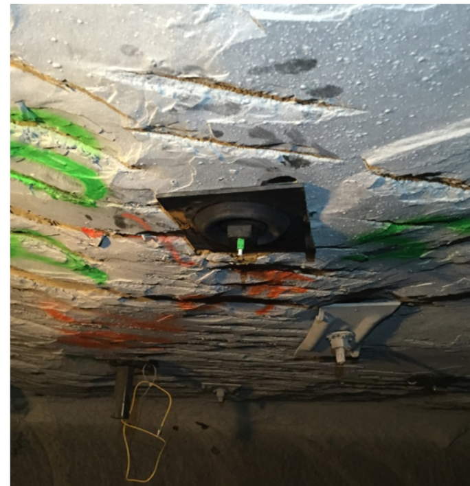
3-groove DOS instrumented bolt installed in shale roof of a coal mine
