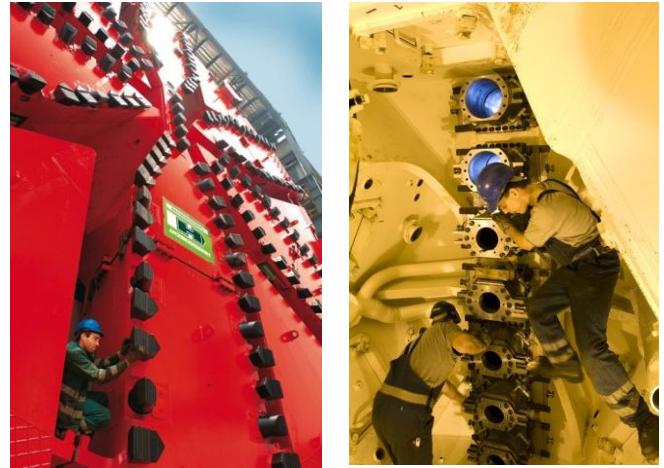
Figure 4. Large diameter Mixshield: accessible cutting wheel in free air for safe tool change
