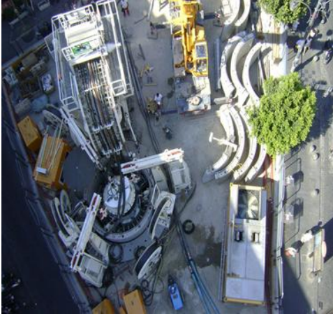
Figure 9. The launch of the Vertical Shaft Sinking Machine VSM9000 using lining segments in downtown Naples
