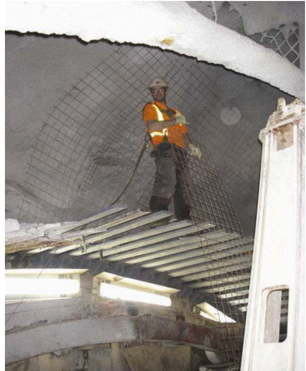
Figure 5. Over-break above the TBM, with room for a worker to stand on top of the roof shield.
