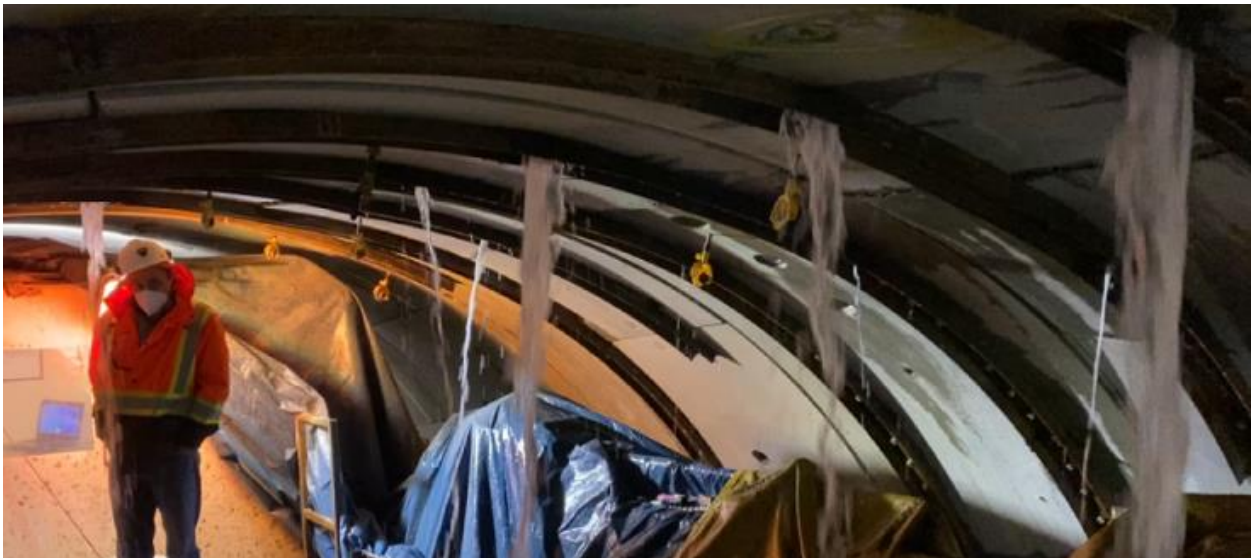
Figure 4. Significant Groundwater Inflow from the Rock Formation above the Tunnel Crown
