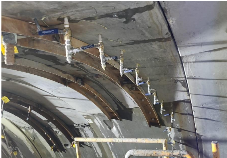
Figure 8. Chemical Grout Collar Radial Injection Ports to Stabilize Ring along with Steel Channels
