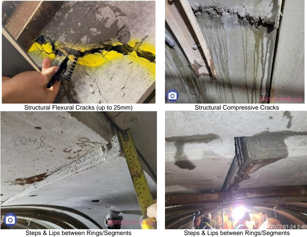
Figure 5. Representative Example of PCTL Damages During Encounter High Water Inflow Events
